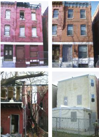
Top row: Front elevation, before and after Bottom row: Rear elevation, before and nearly complete
