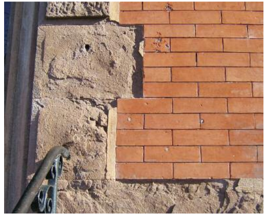
Top: Brick damaged by dripping air conditioner Bottom: Deteriorated brownstone trim
